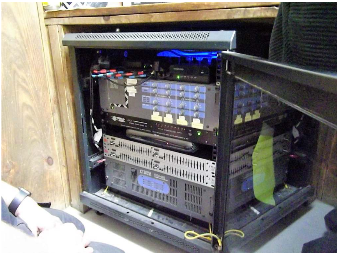
Figure 9: Amplifier rack in Manager's Office with Formula Sound AVC-2 limiter
